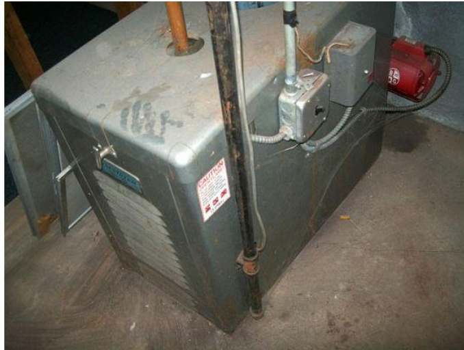
Very old heating system boiler and associated components
