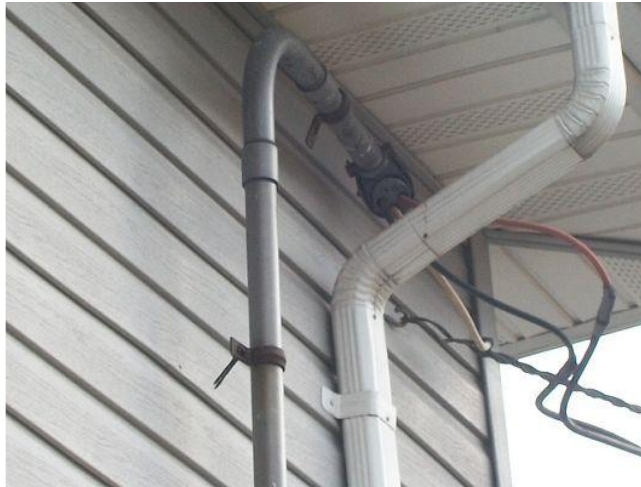
Service entry conduit detached from the home
