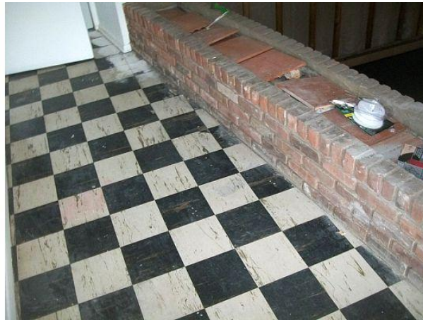
Old floor tile likely contains asbestos
