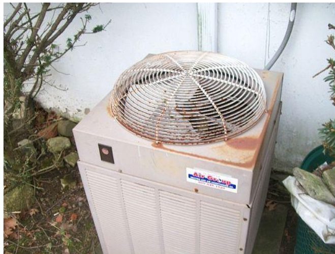
Aging AC equipment
