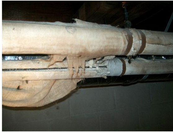
Pipe insulation likely to contain asbestos
