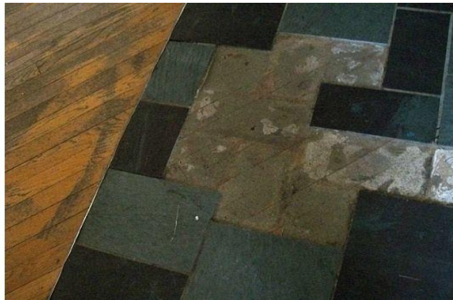
Loose slate in entry hall
