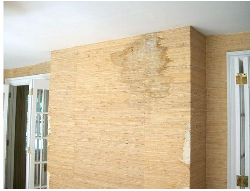
Leakage staining around chimney on the interior
