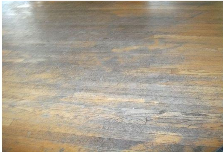
Worn & stained wood finish flooring
