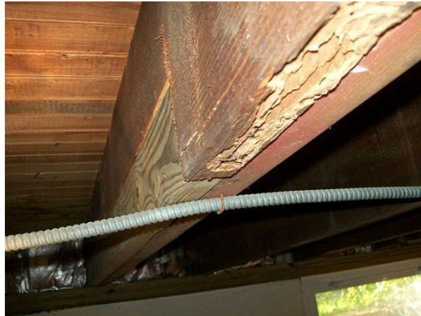
Termite damage to a floor joist with only partial & inadequate repairs.
