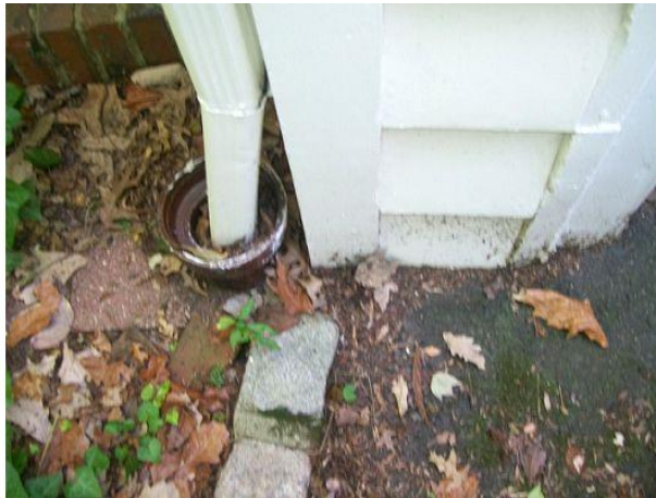
Old clogged underground clay pipe
