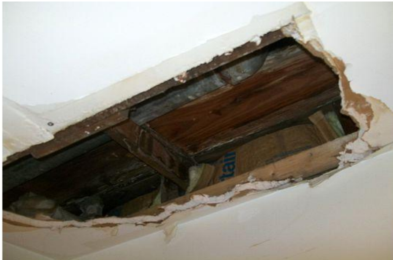
Hole in kitchen ceiling
