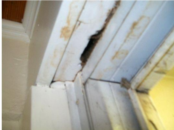
Water and ant damage to perimeter wood at enclosed patio room
