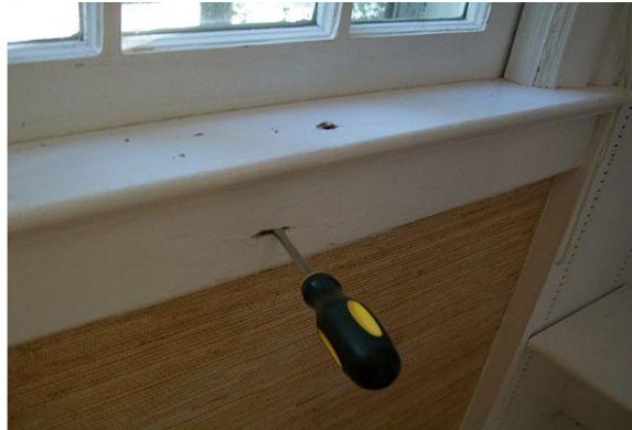
Termite damaged interior trim
