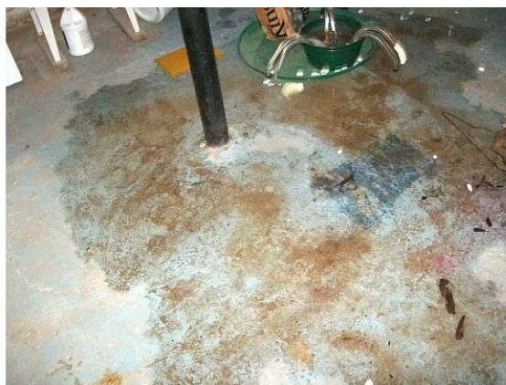
Water on the basement floor
