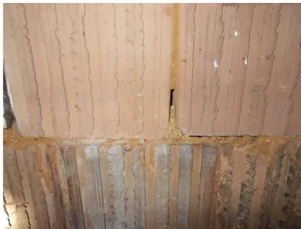
Gaps and soft mortar in terracotta block
