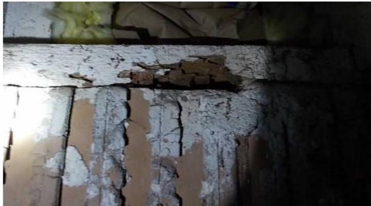
Powder Post Beetle damage to sill plate
