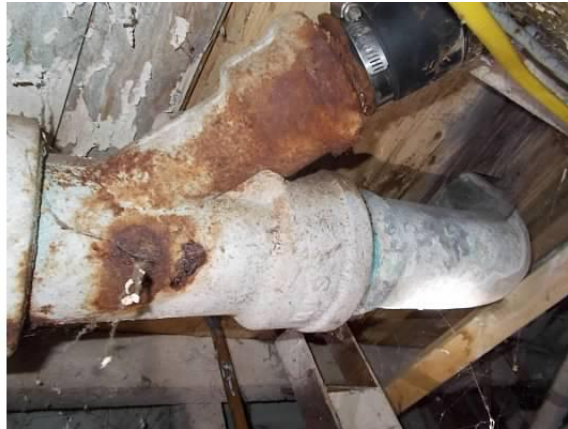
Badly corroded and leaking drain pipe
