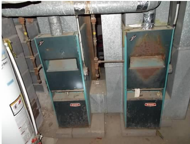
Two of the four heating systems
