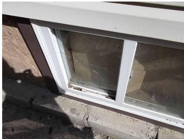
Broken basement window glass
