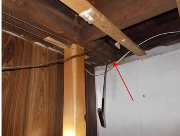
Probe easily penetrates end of Termite damaged beam
