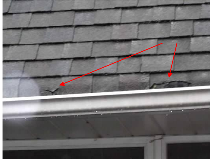
Worn and cracked lower sections of shingles
