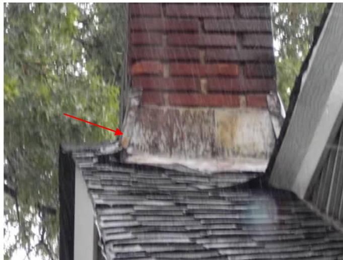
Poorly installed chimney flashings
