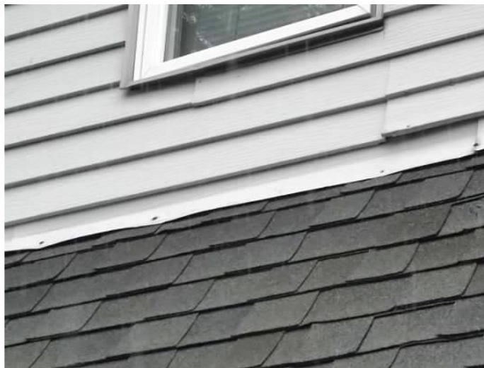
Poorly attached lower section of siding
