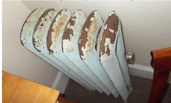
Peeling paint on radiator
