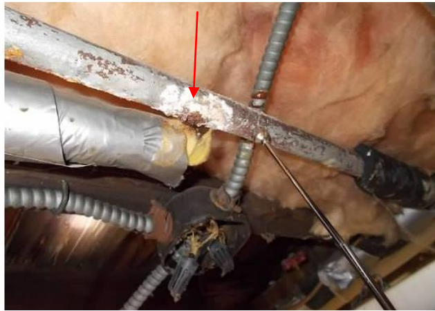
Corroded and leaking old iron water supply pipe
