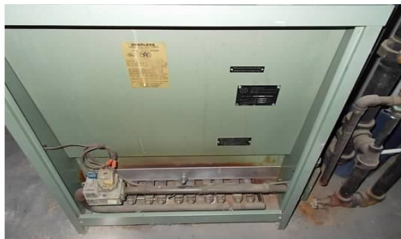
Aging steam heating system
